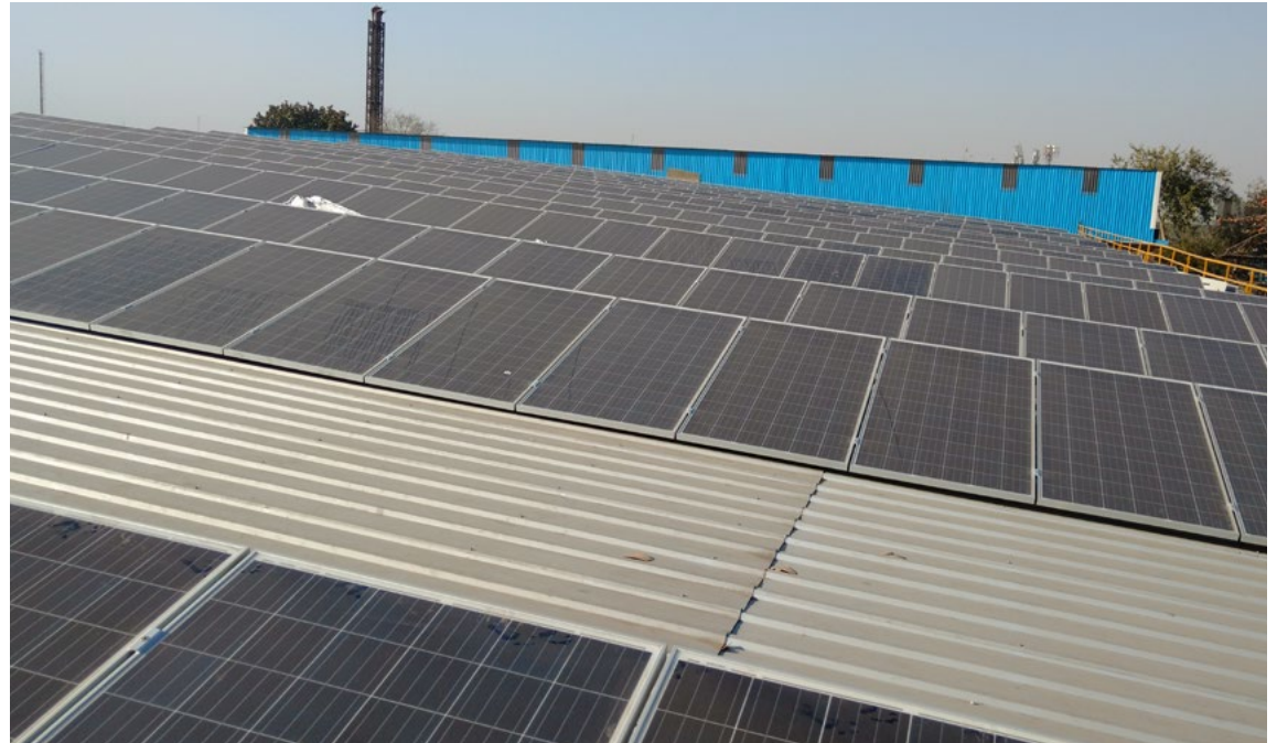
Solar power system installed August 2016, in Pune, Maharashtra, India
